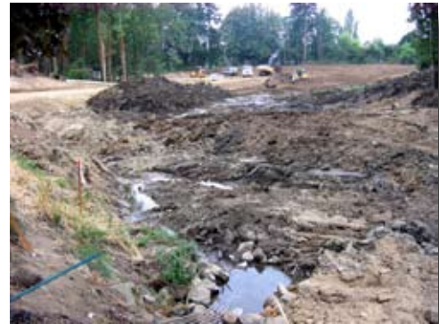
Existing pipe discharging into the Encore facility.
