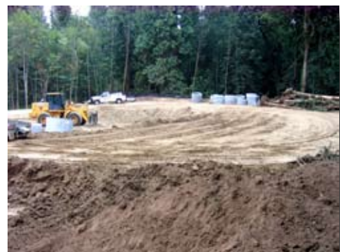
Staging for construction of the pond outlet that controls the rate of stormwater released.
