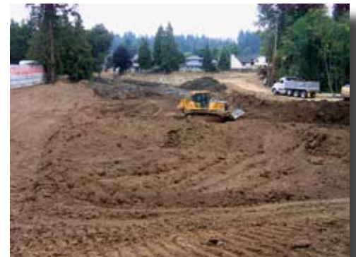
Excavation of the new pond where water will flow from the top of photo to the right.
