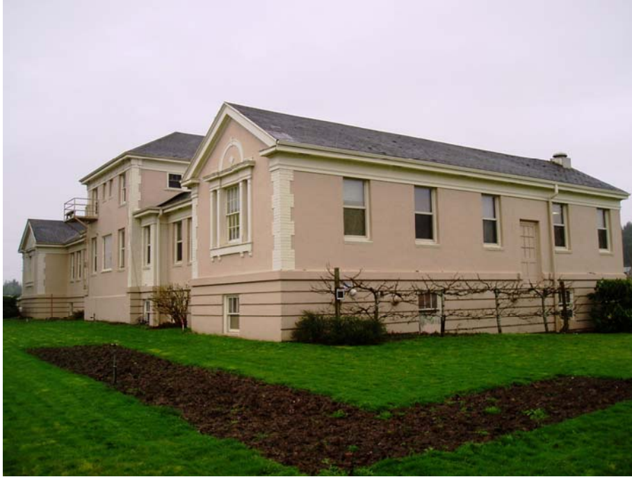
Figure 8. Clark County Poor Farm Main Building, view across the north elevation (left) and west elevation (right). The view is to the southeast.
