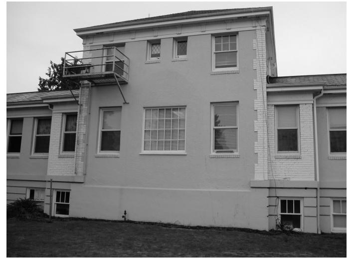
View of Clark County Poor Farm Main Building, view to the south taken 2/26/2010
