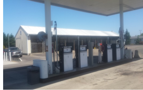
Photo 5: Operations Center Fuel Dispenser
