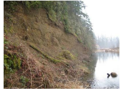
Unstable soils show recent erosion along the south bank of Manley Creek.
