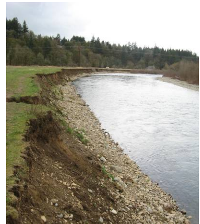
Streambank erosion on the site adjacent to the East Fork Lewis River.
