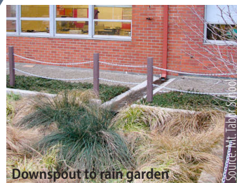
Downspout to rain garden
