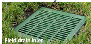
Field drain inlet
