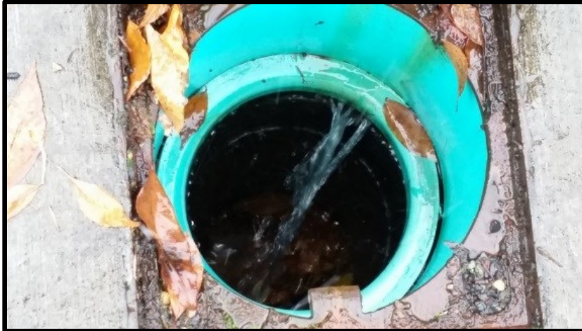
Figure 15. Close-up image of subsurface seepage under a south curb inlet between green reducer and black vertical pipe (taken during heavy rain event on 10/22/2014)
