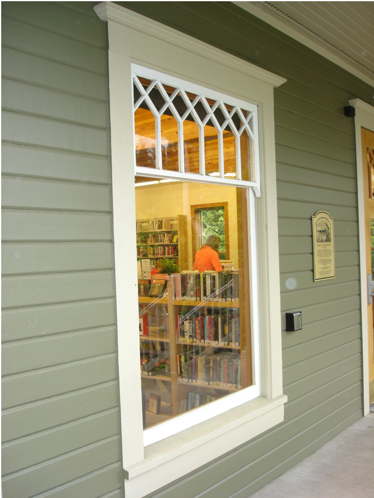
WA_Clark County_Zener House_06 Detail of west façade showing original window Date of photo: 6/16/2017 Photographer: Holly Chamberlain
