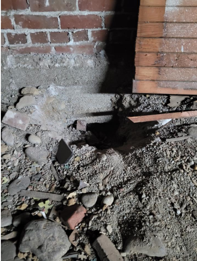
NO FOOTING UNDER BEARING WALLS
